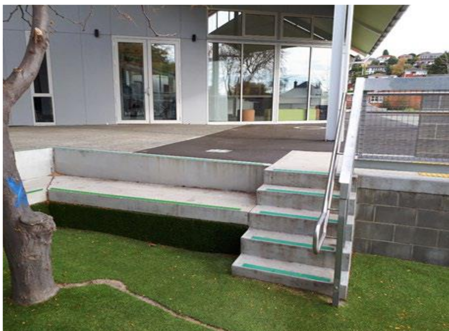
Figure 5: The top of the concrete ramp depicted from the sunken sitting area.
