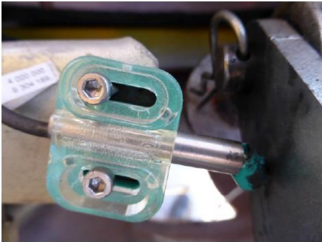
Figure 38 Airmaxx 360 Damaged proximity switch due to contact with R-Clip (P1010459.JPG)
