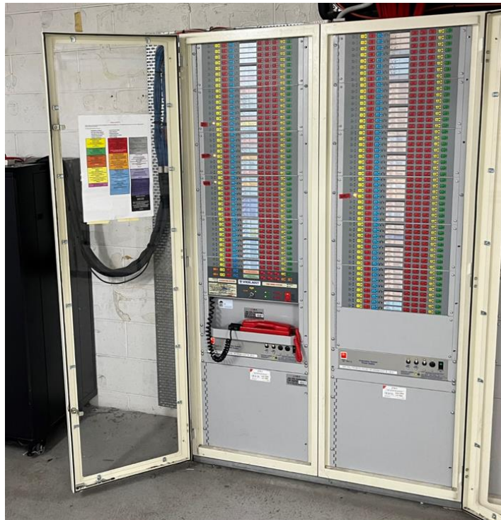
Figure 15: EWIS panel located in the Fire Control Room
